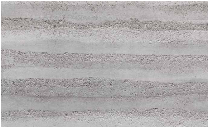
RAMMED EARTH WALL LIGHT GREY*
